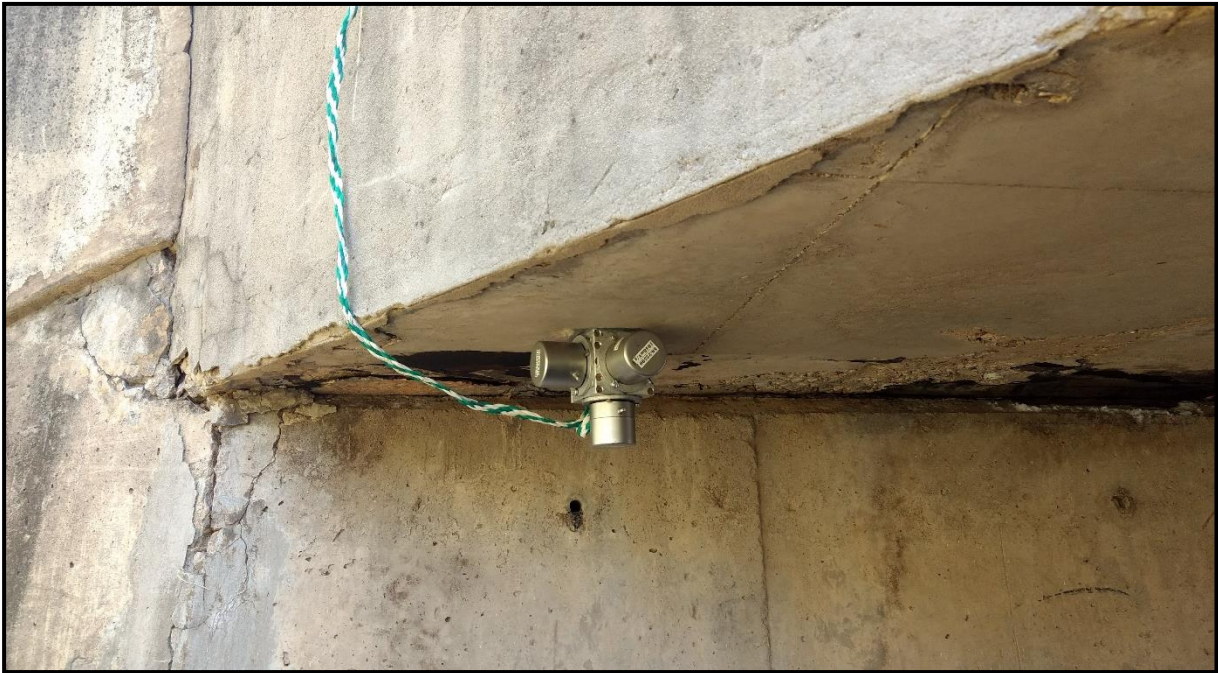
Figure C-1: Photograph of the Three Seismic Accelerometers on the Measured Bridge (safety cord also visible)
